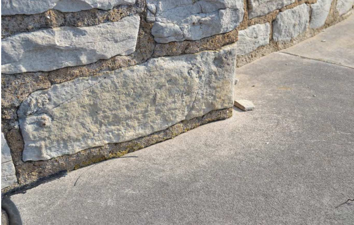
Photo No. 3 Typical juncture of low coping and high parapet wall. See masonry restoration note 4H – cut out mortar at juncture of wall and coping to \frac{3}{4} " to allow installation of sealant.
