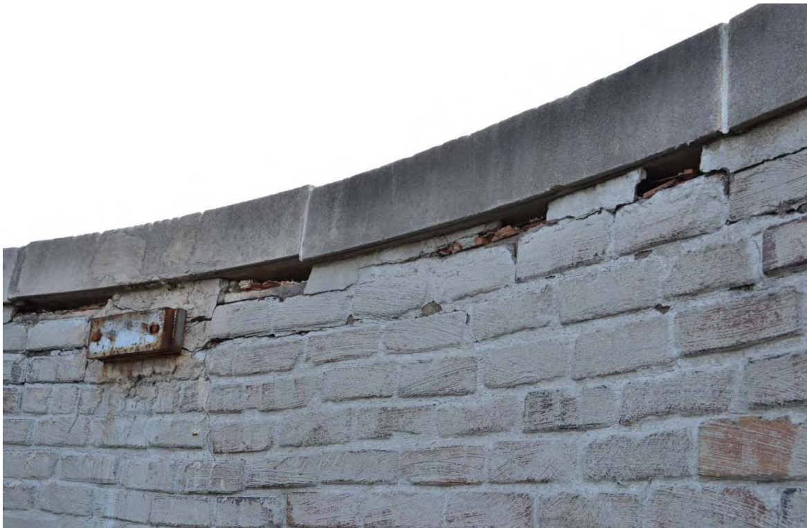
Photo No. 6 Displaced stone coping at parapet B, east side of building. Remove coping stone and five courses of brick. Reconstruct – see notes 4B and 4K
