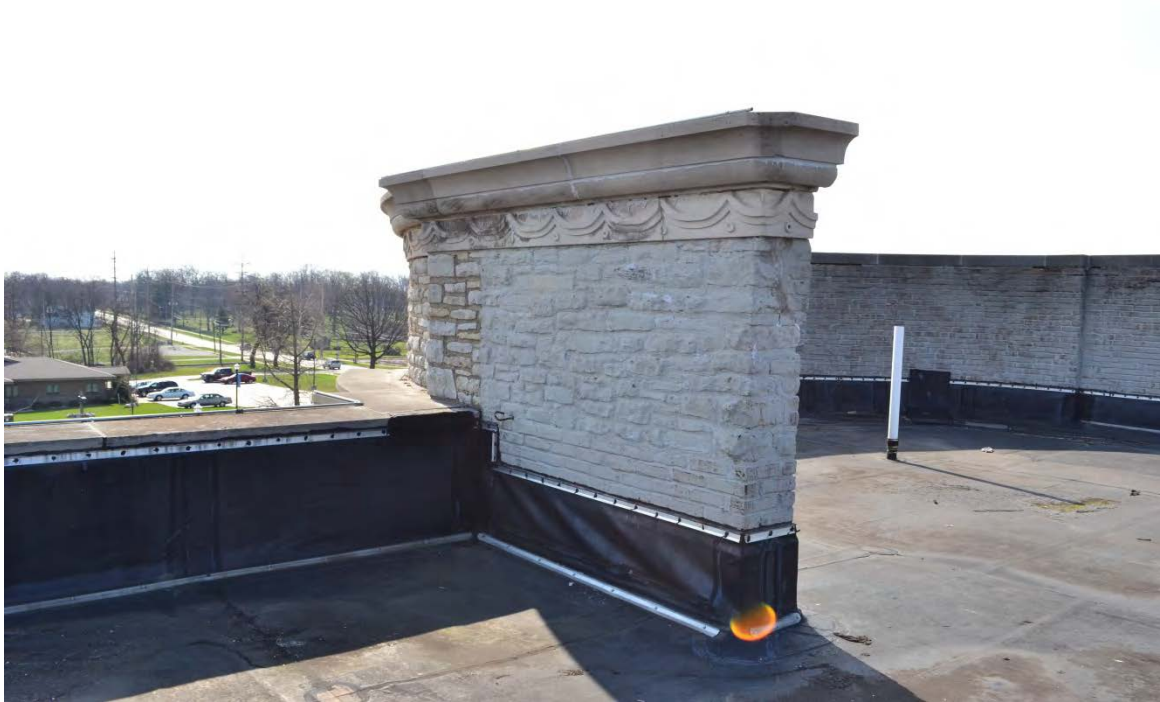
Photo No. 7 North side of wall in photo no. 6. Replace all coated stone with new stone when reconstructing this wall. See notes 4B, 4J and 4K
