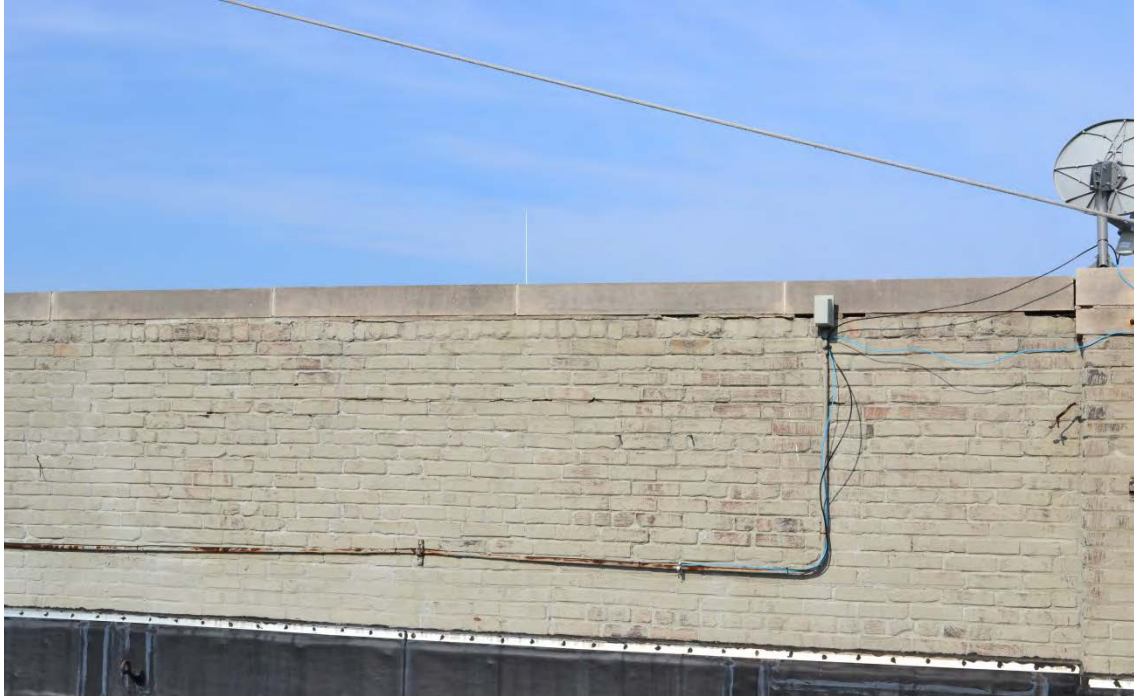
Photo No. 13 West wall at parapet B on west side of building. Remove and re-set stone coping and five courses of brick note 4A- 4K. Communications wires to remain – Coordinate with owner.
