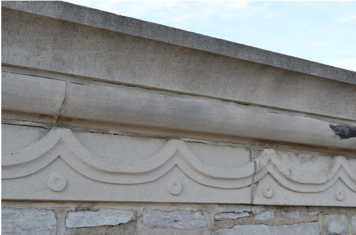
Photo No. 11 Close-up of carved stone cornice and coping typical at Parapet B. Notes 4B, 4G and 4K
