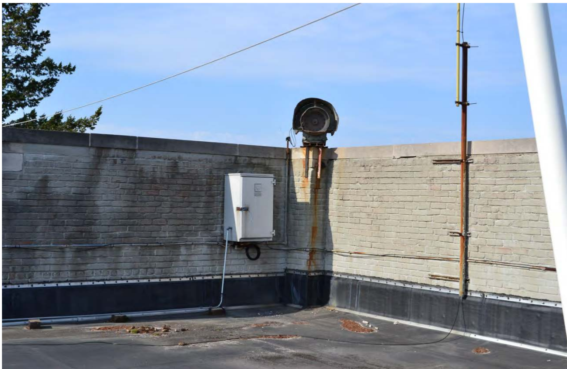
Photo No. 14 Southwest corner of parapet B on west side of building. Electrical to remain – coordinate with owner.
