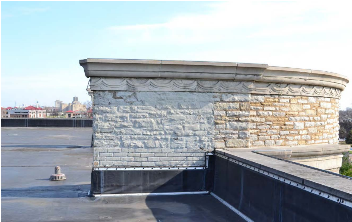
Photo NO. 2 South elevation of Parapet B on east side of building. Profiled stone to be removed and reinstalled. Refer to masonry rehabilitation notes 4A-4K.
