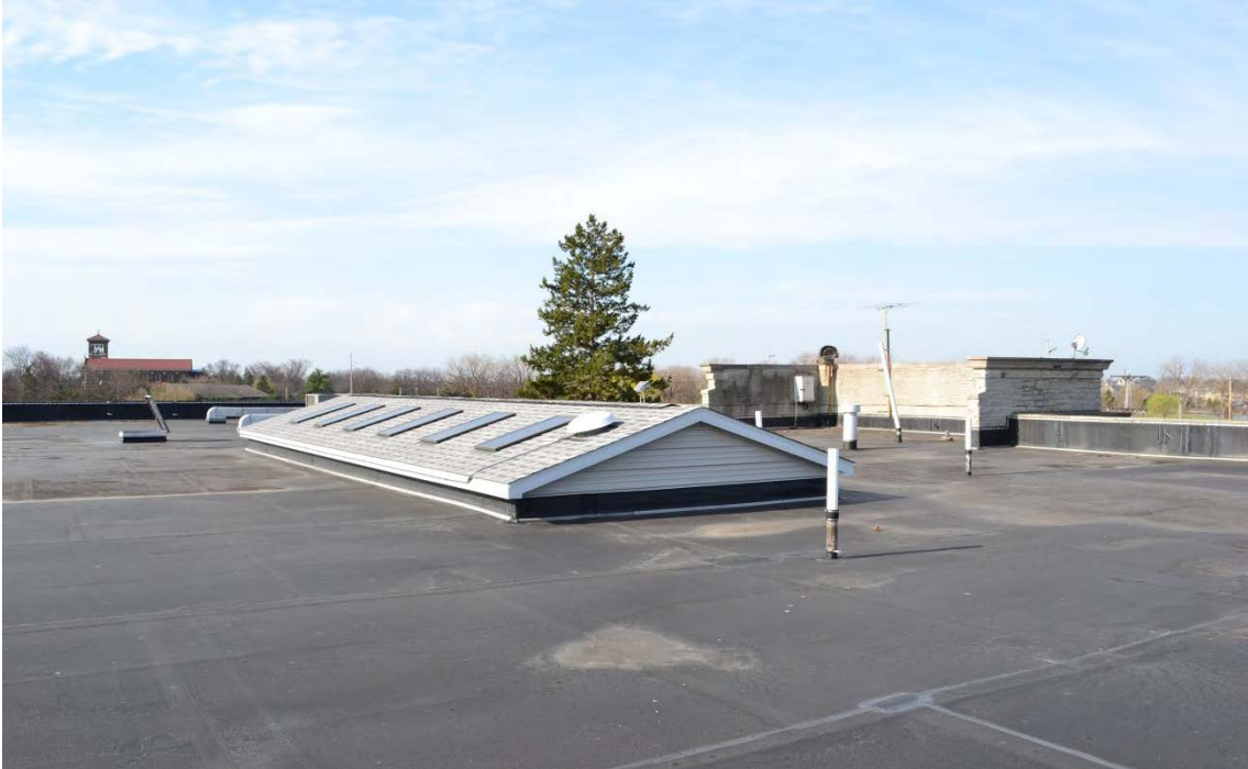
Photo No. 9 Parapet B on the west side of the building. See Notes 4A-4K
