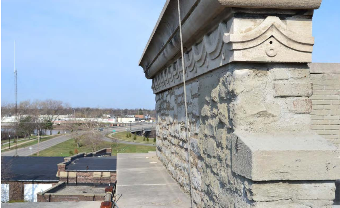
Photo No. 15 South wall of parapet B on west side of building. Cut in sealant joint between lower coping and upper parapet wall – see Note 4H.
