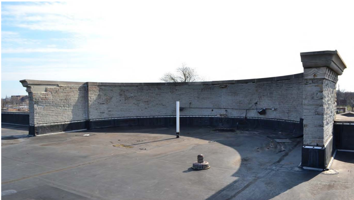
Photo No. 4 West side of parapet B on east side of building. See masonry rehabilitation notes 4A-4K
