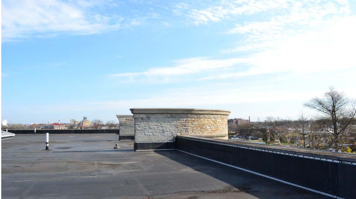
Photo No. 1 Parapet A – low parapet – cut out joints in coping and install new sealant. Parapet B – tall parapet at center of east elevation. See masonry rehabilitation notes 4A – 4K.
