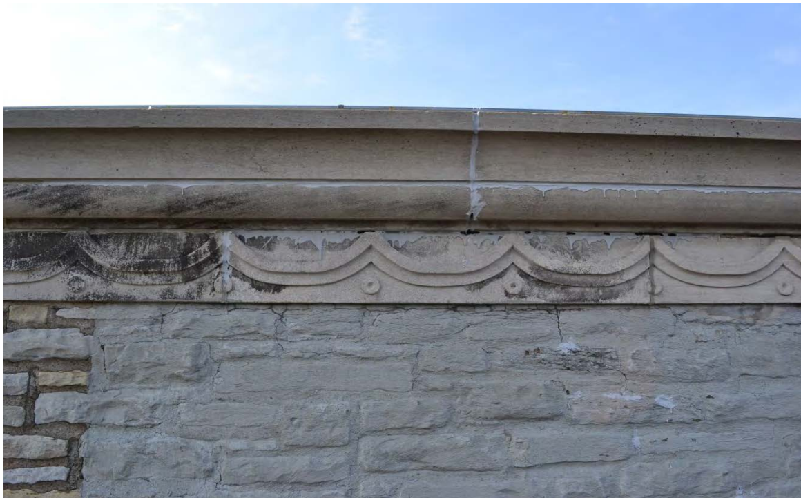
Photo No. 8 Close-up of photo no. 7. Remove sealant from cornice and coping before reinstalling.
