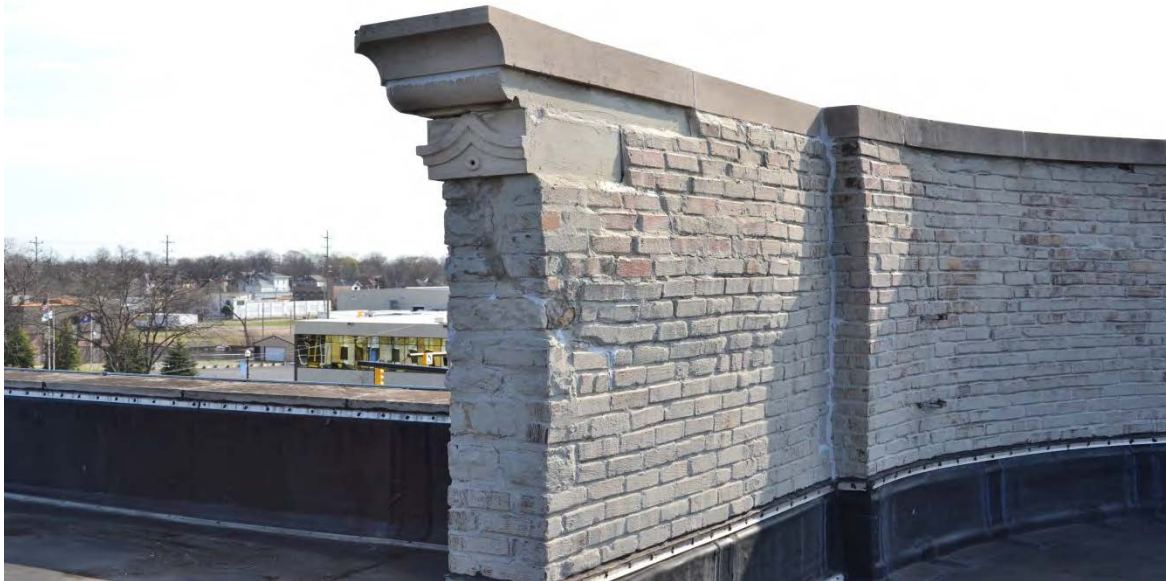
Photo No. 5 Northwest corner of parapet B on east side of building. The section of wall from the offset to the west is to be removed and reconstructed from the roof flashing to the Top of the wall. Notes 4B, 4J and 4K
