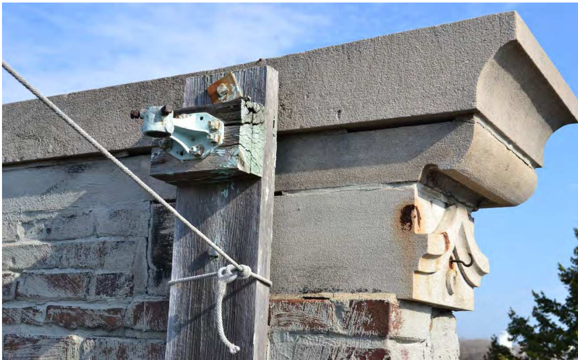
Photo No. 12 Wood support and "J" hook -- see note 4A. Note: the rope is currently supporting an extension on a vent stack. The extension will be re-supported or removed.
