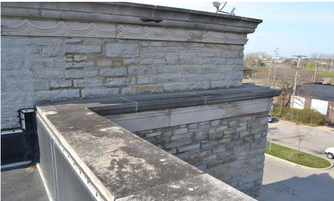
Photo no. 10 Parapet A in foreground -- see notes 3A-3B. Parapet B beyond – see notes 4A-4K.
