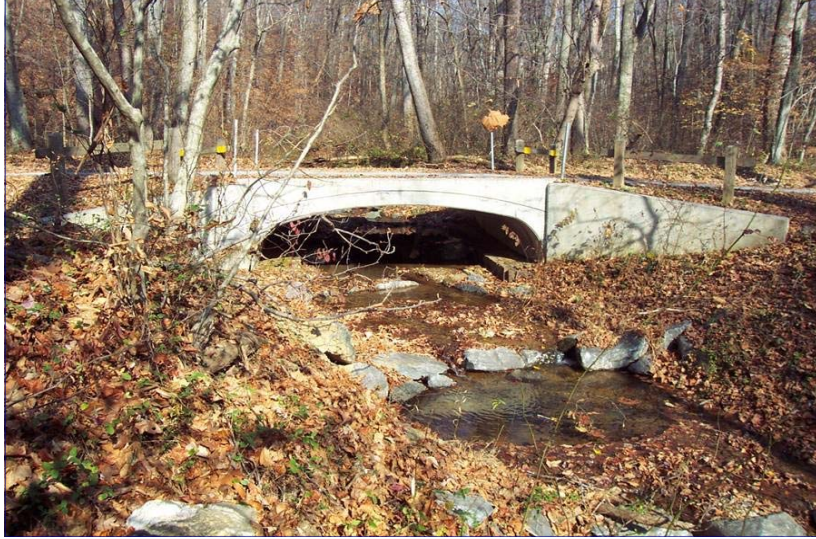
IMPACT 1 - Conspan with a natural stream bed and only temporary impacts during construction.
