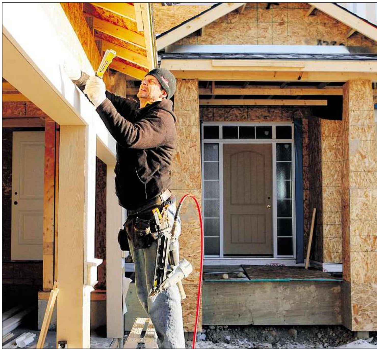
Steve Plett works at an under-construction Calgary home. A pause in new construction will help manage the supply, says an analyst.
