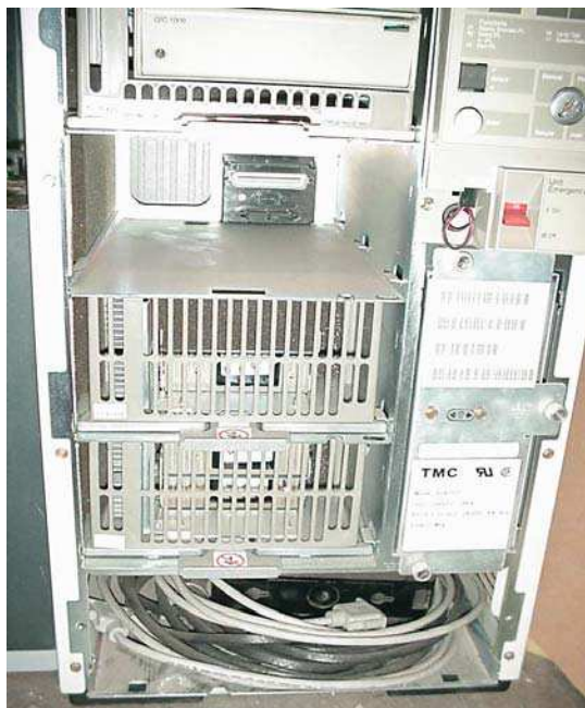
IBM AS/400 System with Drive Bays Exposed
