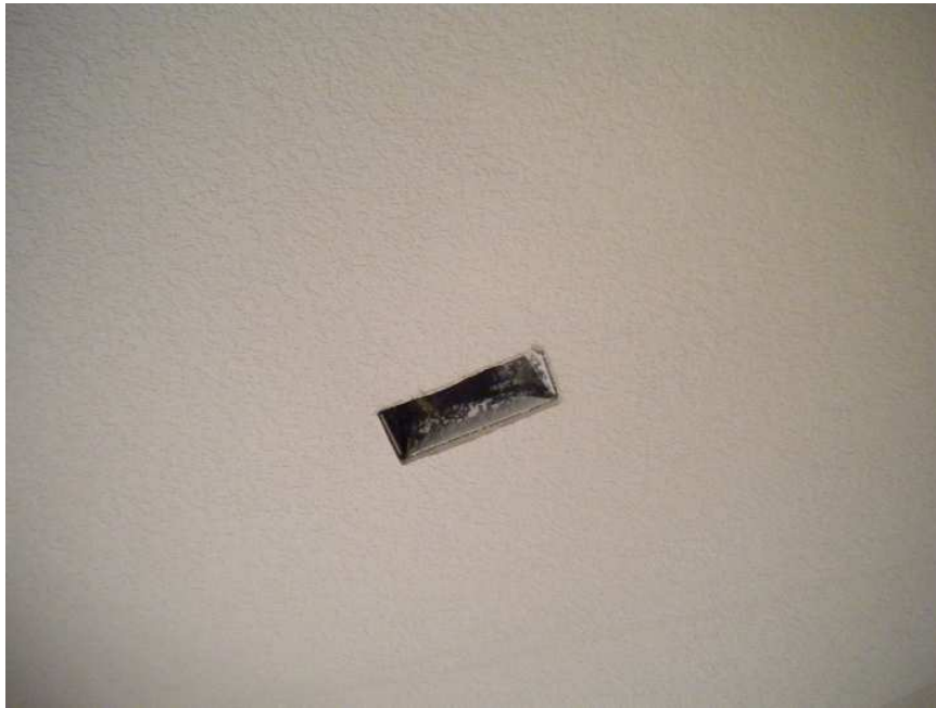
View of Ceiling Vent@ Kitchen
