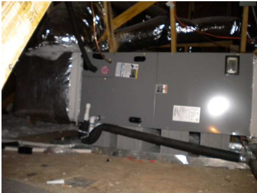
View of Furnace in Attic
