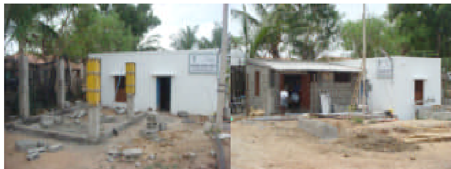
Illustration 5. The different stages of the construction of the main building. An additional, bigger room has been added to the already existing building.
