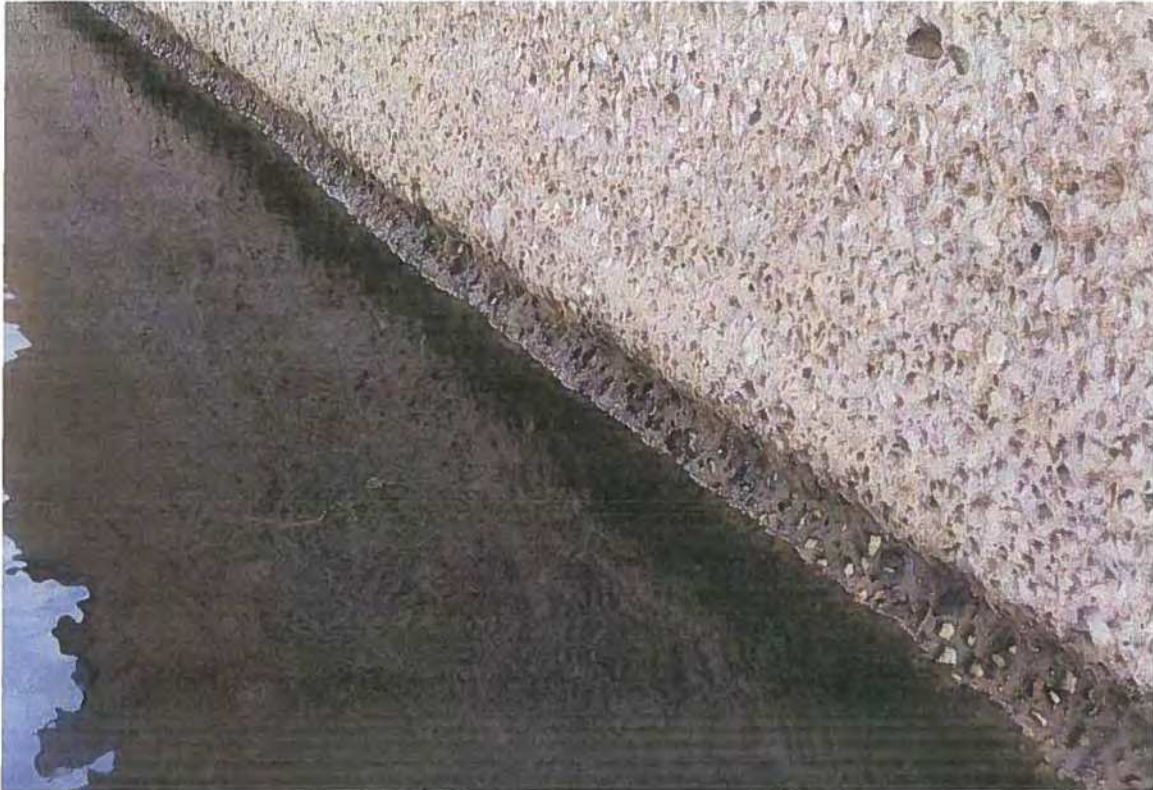
Downstream - South End Wall. Note "Grooved" Channel at Water Surface.
