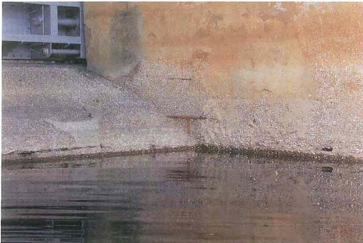
Downstream - North Bay Wall New Spillway. Note Exposed Reinforcing Steel.
