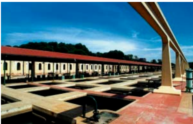
Images of the San Martín water treatment plant, Buenos Aires, Argentina. All pictures courtesy of Ondeo Services / Thierry Duvivier.
