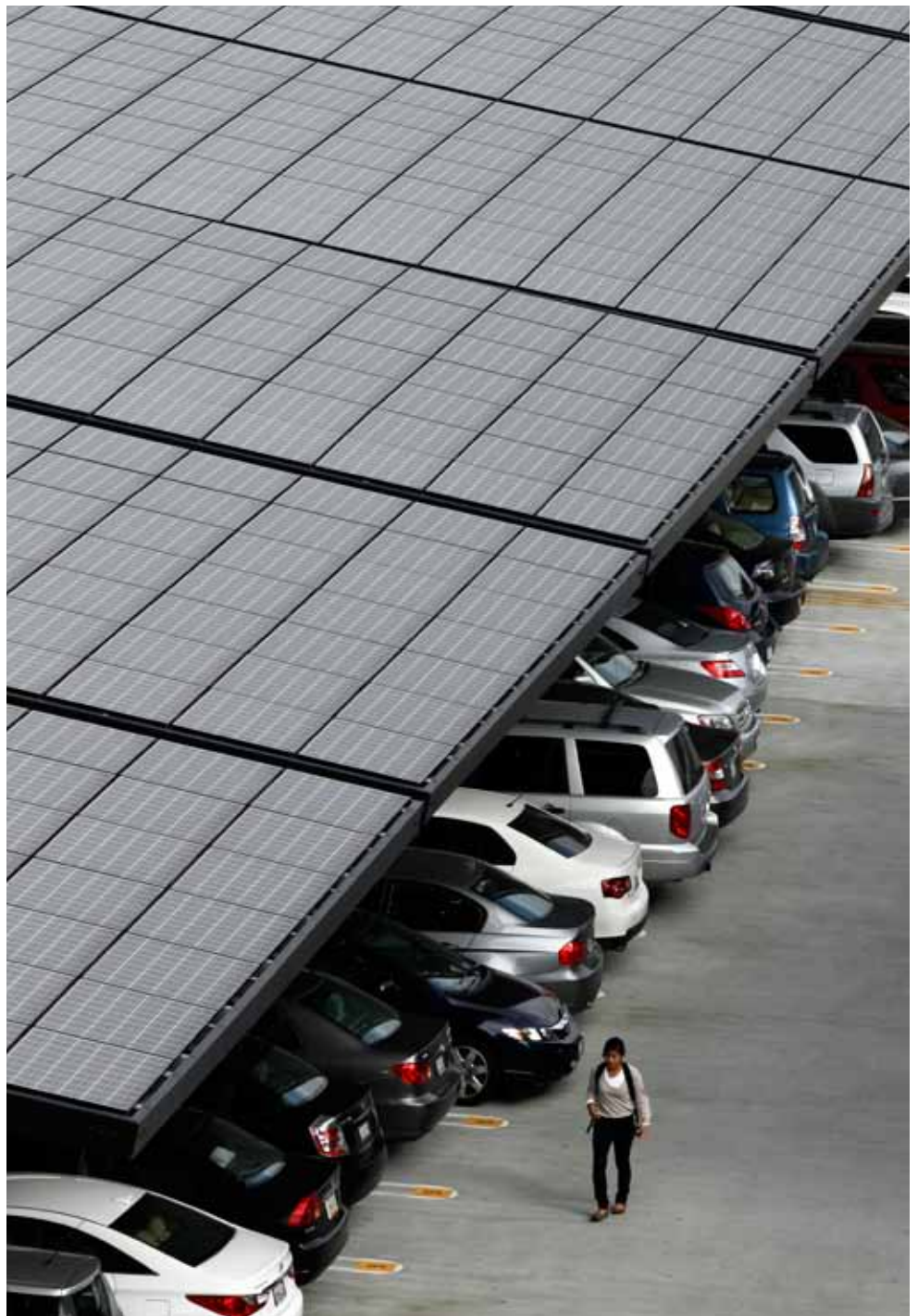
DOUBLE DUTY: A parking structure at the University of San Diego California uses innovative solar trees to collect renewable energy from the Sun February 8, 2011. REUTERS/MIKE BLAKE
