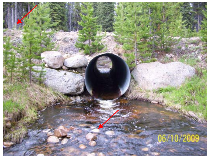
Photo 1: Outlet of old Red2 culvert showing no embedment, a 3 cm outlet drop, and a culvert that does not maintain natural stream width. At low flows, water depth would prevent upstream fish passage whereas the natural channel was always passable.
