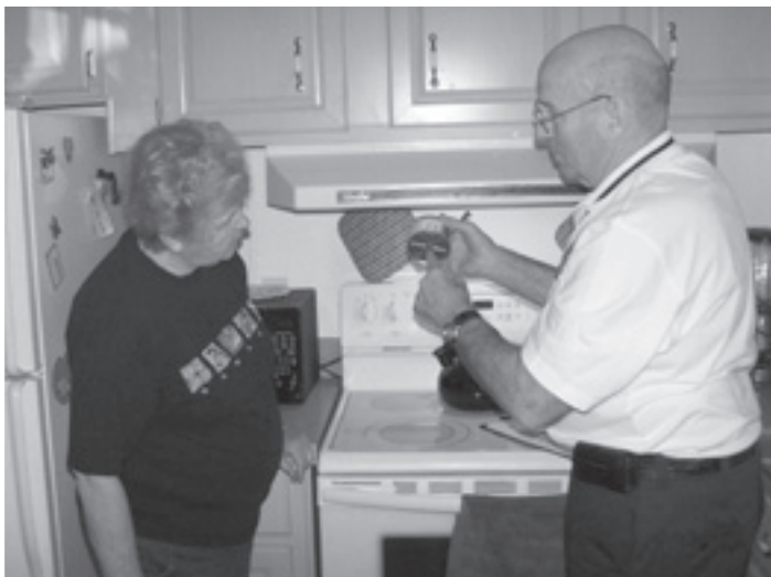
Fire Inspector Charlie Bracewell installs an automatic fire extinguisher above the stove.
