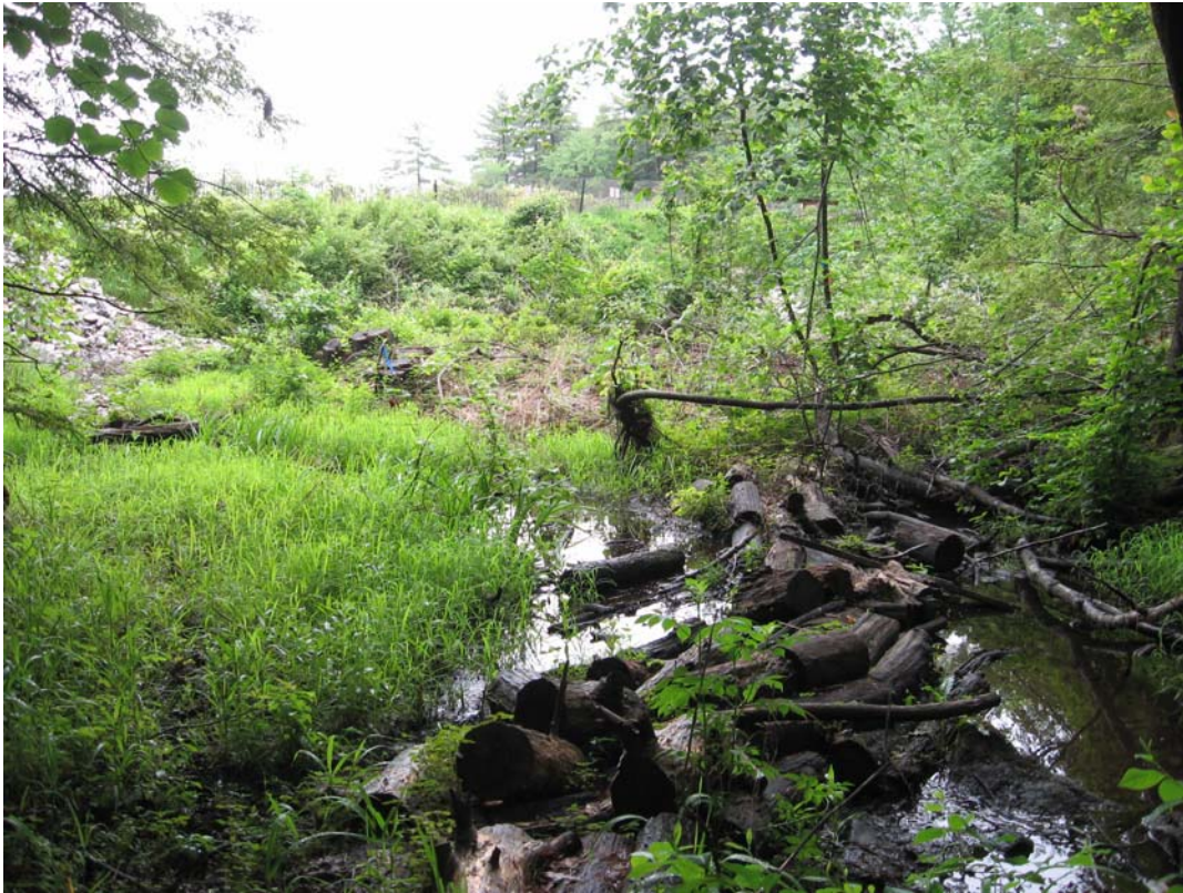
Photo 009. Cut timber placement at apparent old spillway outlet
