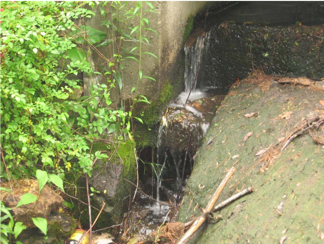
Photo 004. Spillway outlet undermining
