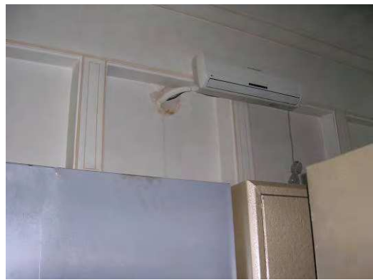
Air conditioning units fitted in some rooms
