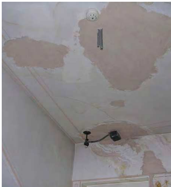
Ceilings with sprinkler systems
