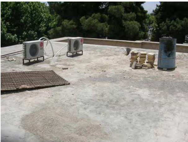
Water proofing being done, however no thermal insulation
