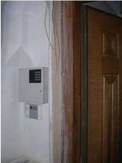
Doors fitted with alarm system
