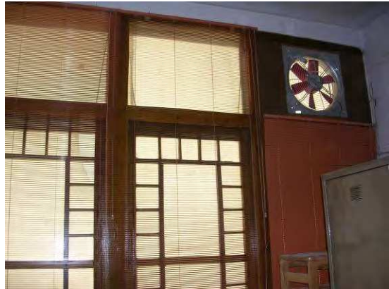
Only one room has a ventilator for air circulation
