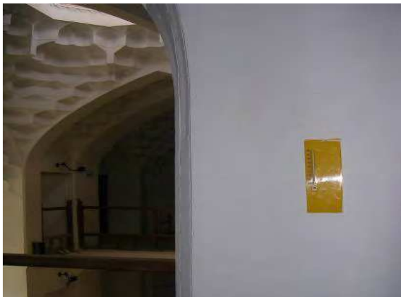
Parts of walls are not plastered or painted
