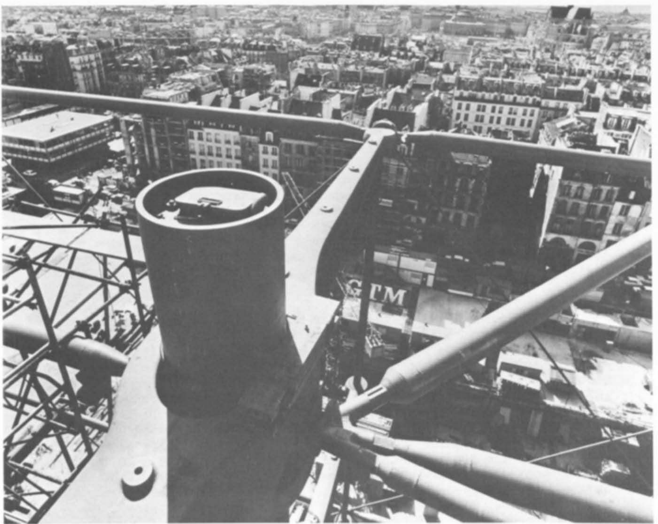
Figure 7—Structure at the top of the Beaubourg Centre in Paris, showing cast steel nodes (Courtesy of Ove Arup and Partners).
