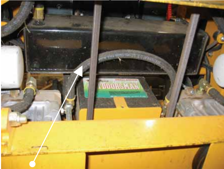
Hose routed horizontally below the hydro tank
