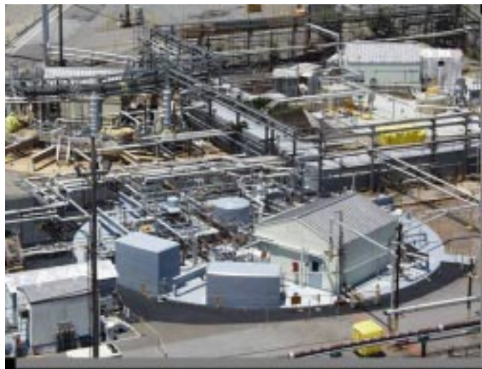
Highly radioactive waste resulting from reprocessing spent nuclear fuel is stored in two tanks farms at SRS.
