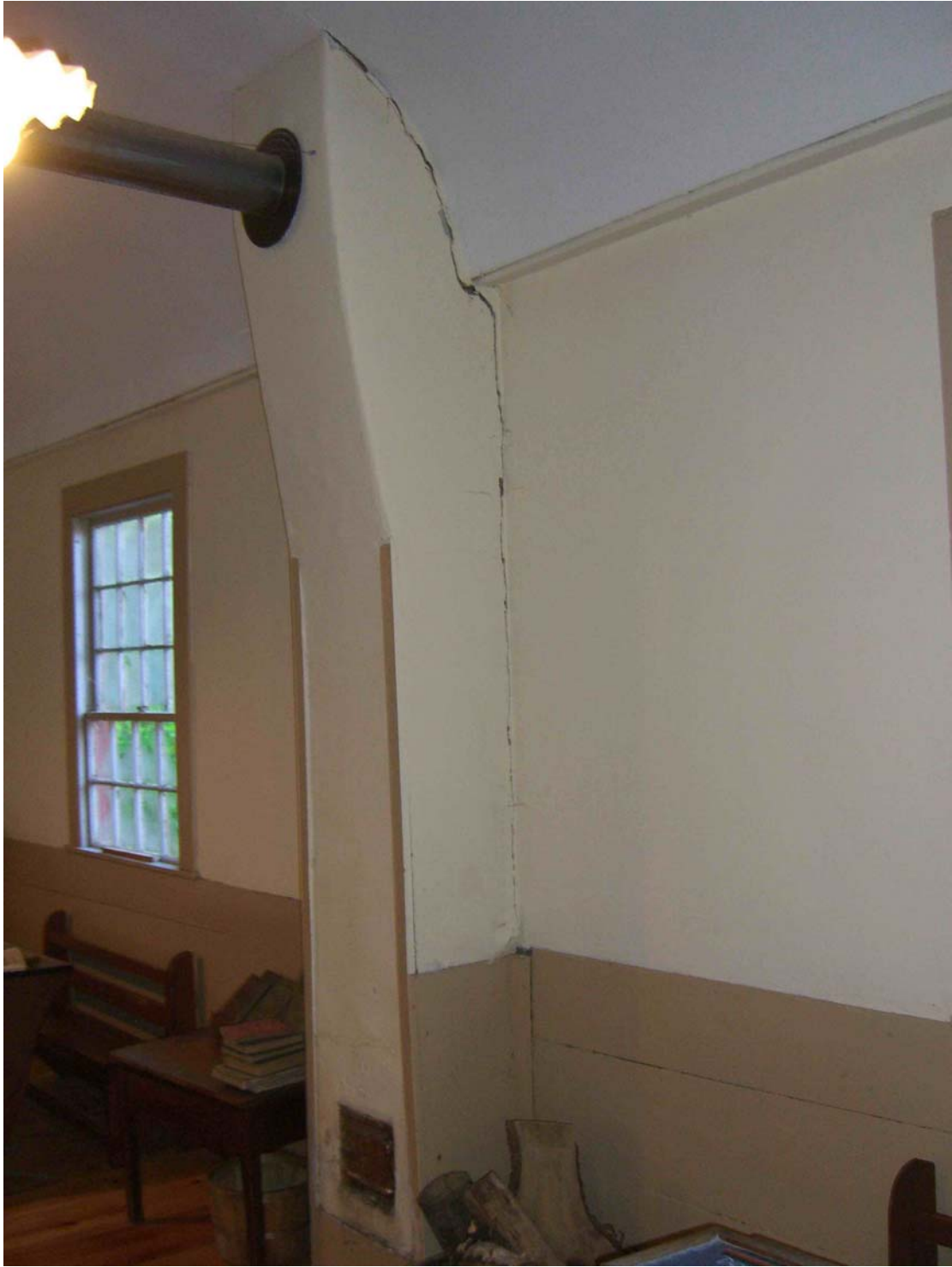
Picture #4 – Chimney separation
