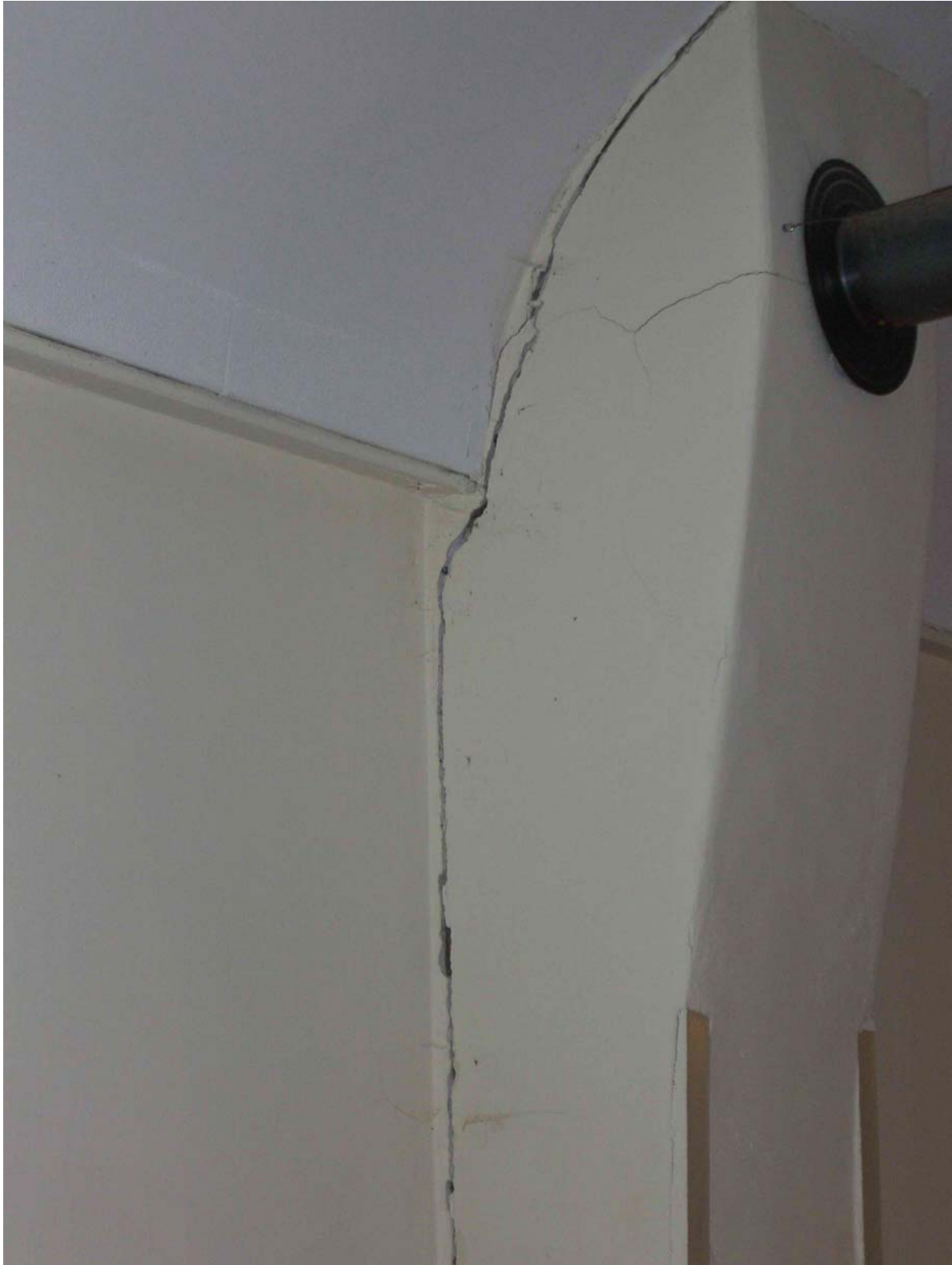
Picture #5 – Chimney separation
