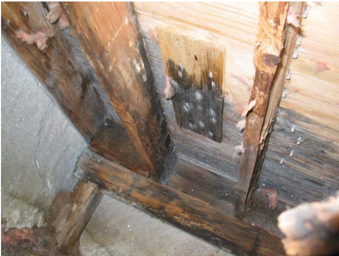
Picture #1 – Rotted beams and supports
