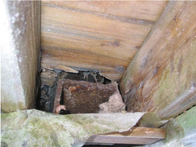
Picture #3 – Rotted supports under chimney
