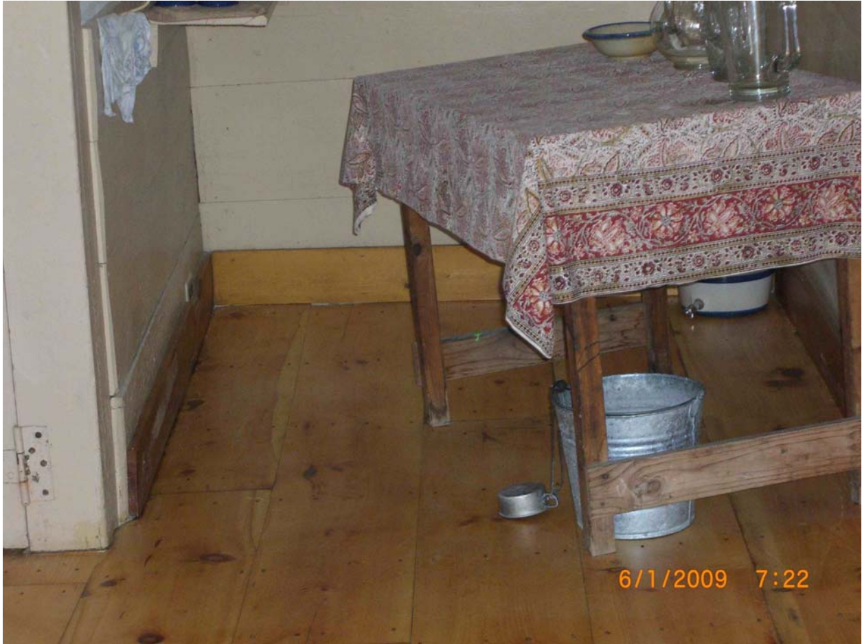
Picture #6 – Sag in floor. Area will support little weight.
