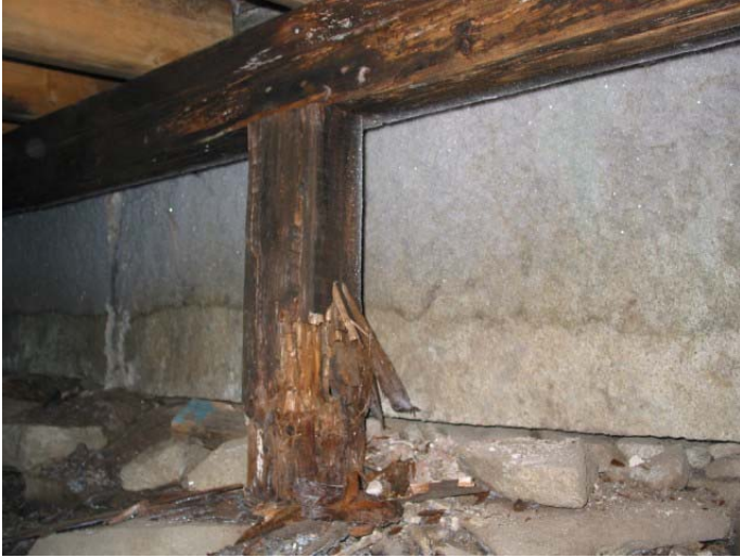
Picture #1 – Rotted support
