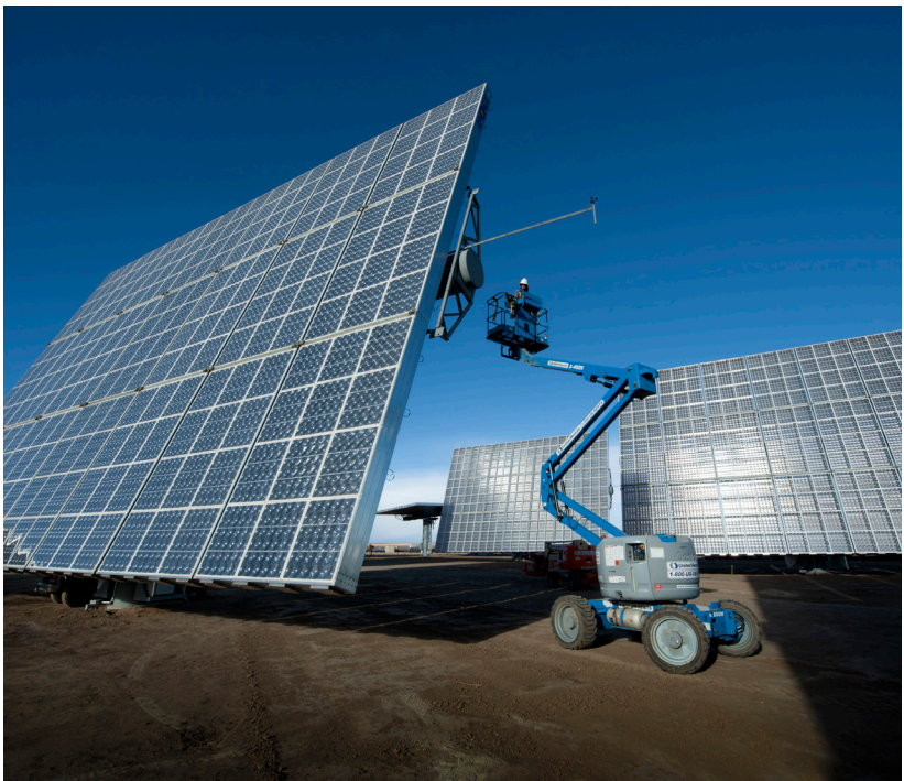
SolarTAC test facility in Aurora, CO (Image courtesy of NREL)
