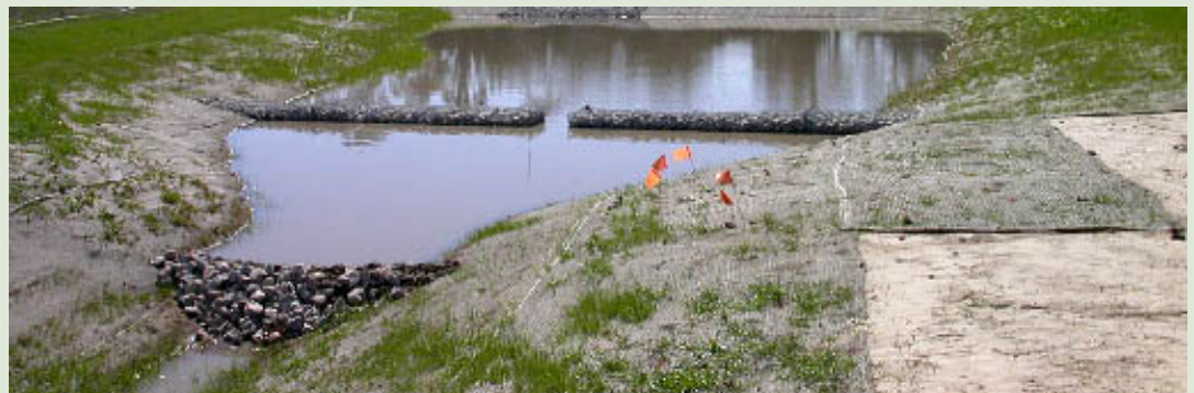
Water retention in the storm water management system following the first winter rains.
