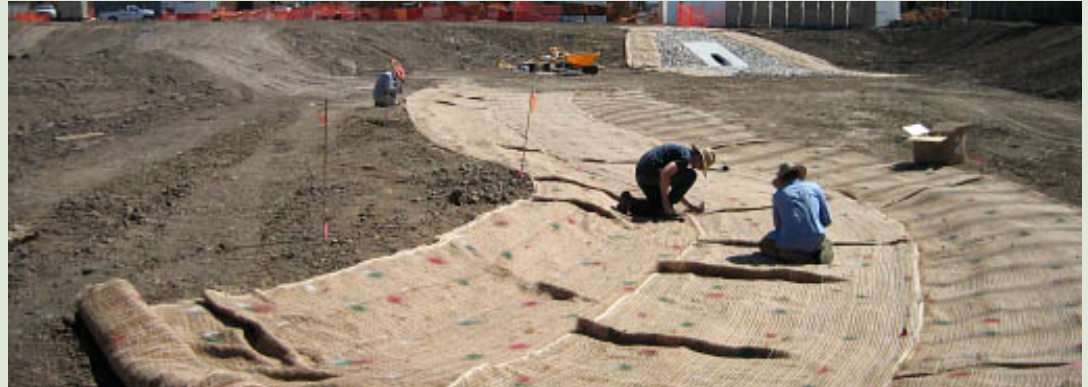
CCBER staff installing coconut netting for erosion control in the storm water management system.
