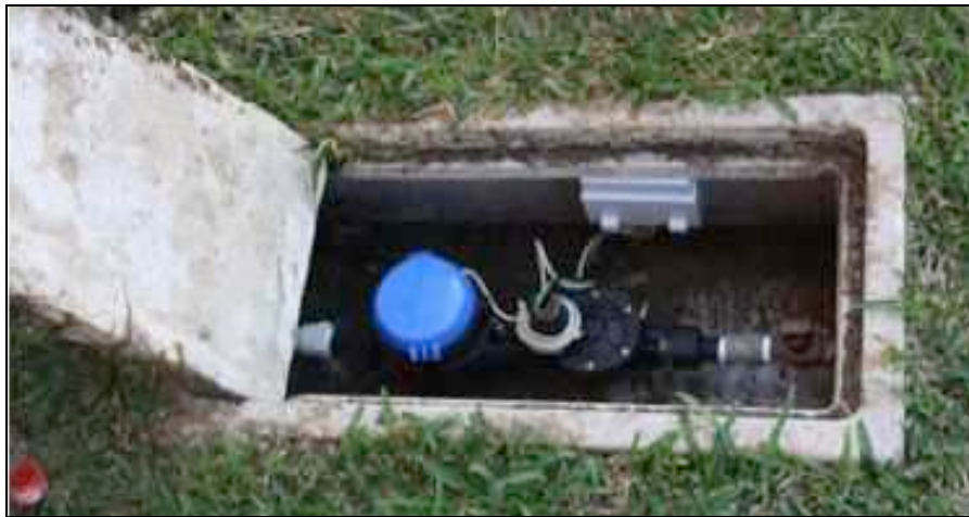
Existing meters with “smart” upgrades provide real-time data
