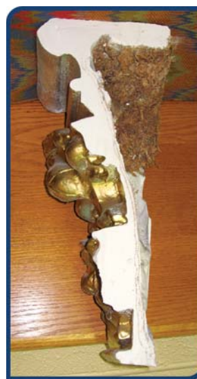
A cross section of the plaster moldings; note the moss and wood chips used as filler.
