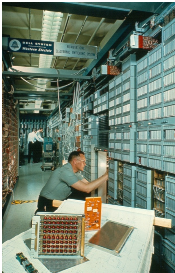
New Jersey Bell Switchman Fritz Blume checks circuit at ESS office in Succasunna, N. J. In foreground are some of the basic units of electronic switching left to right: dual sensor, permanent memory card, ferreed switch array, logic circuit pack (orange) and twistor memory sub-assembly.
