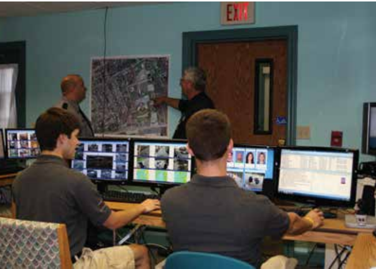
LLWS command center centrally monitors alarms, video surveillance, access control and badging.
