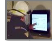
Integrated Emergency Communications Controls
