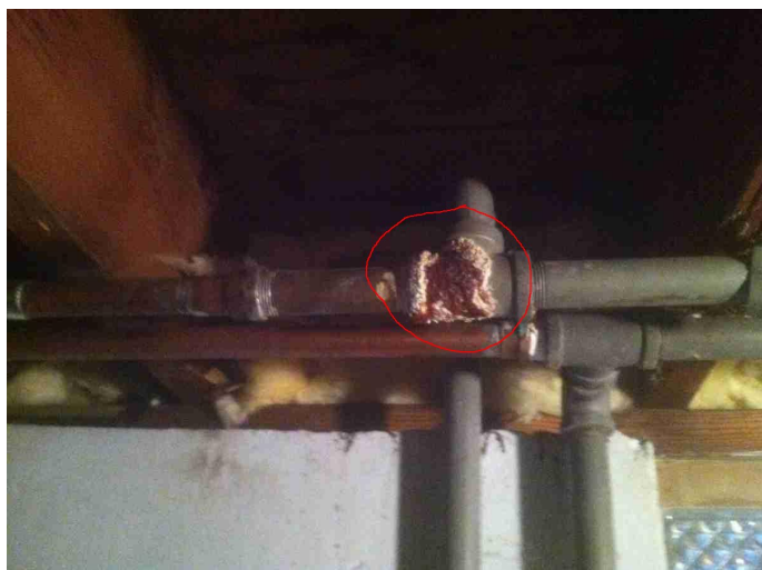
Water Source - CONSIDERABLE DAMAGE / CORROSION / UNSATISFACTORY CONNECTIONS NOTED
