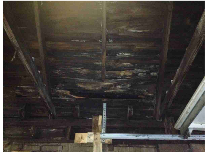
Structure / Attic / Crawl Space & Ventilation - CONSIDERABLE DAMAGE / DECAY / NOTED TO MEMBERS
