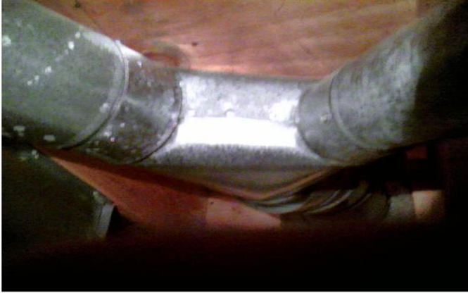
Flue / Vent Pipe - RECOMMEND VENT / FLUE STACKS ARE JOINED WITH A WYE "Y" PIPE
