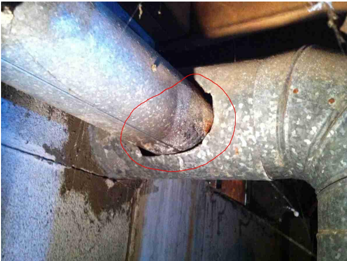
Flue / Vent Pipe - PROPERLY SEAL / JOIN FLUE/VENT PIPE
