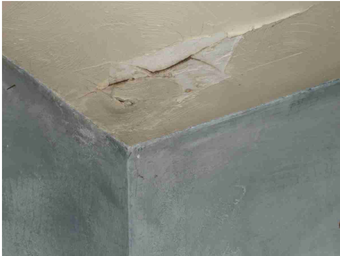
Wall / Ceiling Coverings - WATER / MOISTURE STAINS
