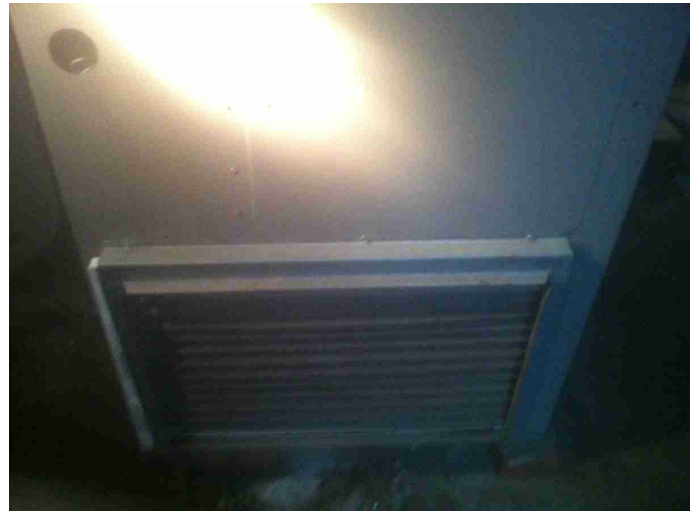
Supply / Return Ducts / Pipes - OPEN DUCTS / RETURNS
