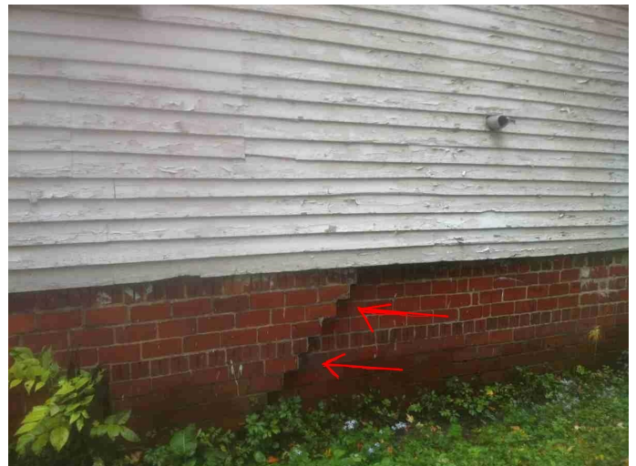
Type / Location / How accessed / Viewed / Condition - Large Vertical / Angled Cracks - EXTERNAL Rear foundation wall
