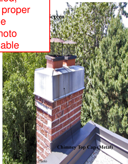
Chimney type / Condition - RECOMMEND INSTALLING A RAIN CAP / SPARK SCREEN
