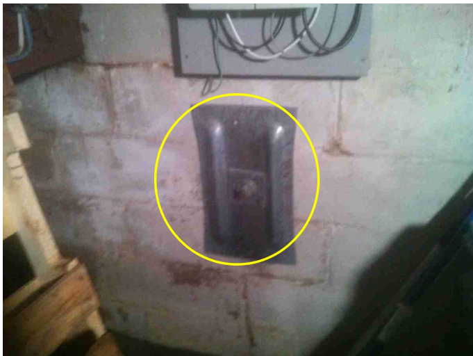
Type / Location / How accessed / Viewed / Condition - Repairs / Patching / Reinforcement - INTERNAL Earth Anchors Noted
