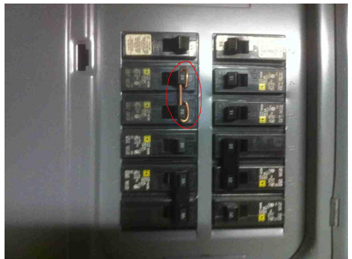
Service Panels / Type / Condition - COUPLER / LINK MISSING FROM 240 VOLT CIRCUIT BREAKER
