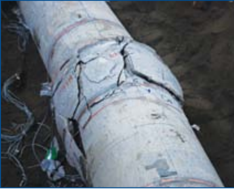
Damage of a concrete pipeline joint incurred during a ground rupture test.
