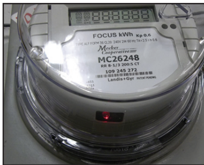
If there is power to the meter, you will see a red light inside the meter, either on the bottom or on the left side, and digital meters will have a numbered display.
