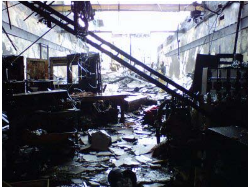
Remnants of fire at 349 E. Main St.
