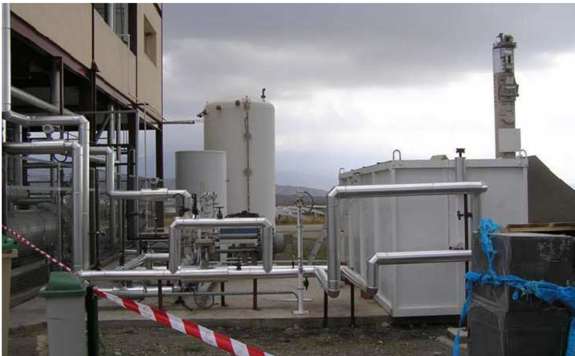
Figure 9. General view of the storage module and the system installed in the PSA DISS plant for its evaluation [23].
