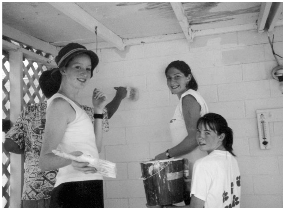
Teens taking part in the PASSPORT national volunteer organization paint the back of one elder's Volusia County home.
