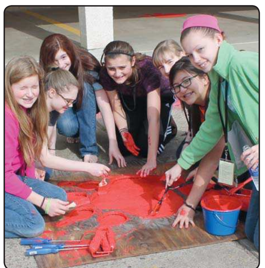
Nearly 300 youths from Sagemont Church volunteered their time Saturday, Feb. 8, to make renovations to Thompson Intermediate. Improvements included painting and adding a sprinkler system to the school's football field. Pictured above painting a Thompson Lion's paw are, left to right, Ellie Martin, Olivia Niemeyer, Olivia Simmons, Bethany Anders, Samantha Smith, Ally Garcia and Ashleigh Thompson. See related photos on Page 5A. Photo by Marie Flickinger
