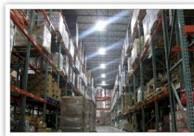
Energy Efficient Lighting
