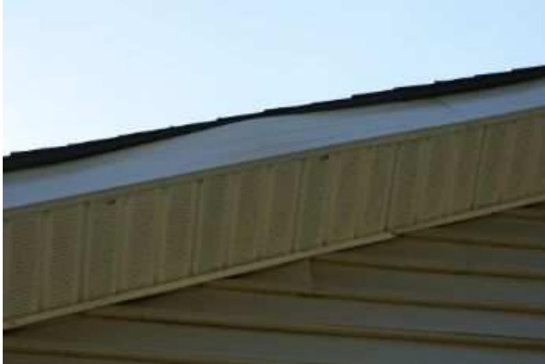
In the rear of house the facial needs to be secured to prevent water intrusion.
