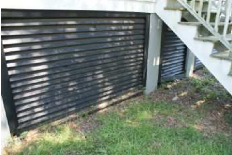
The Lattice under the front porch near the ground has some rotted sections.
