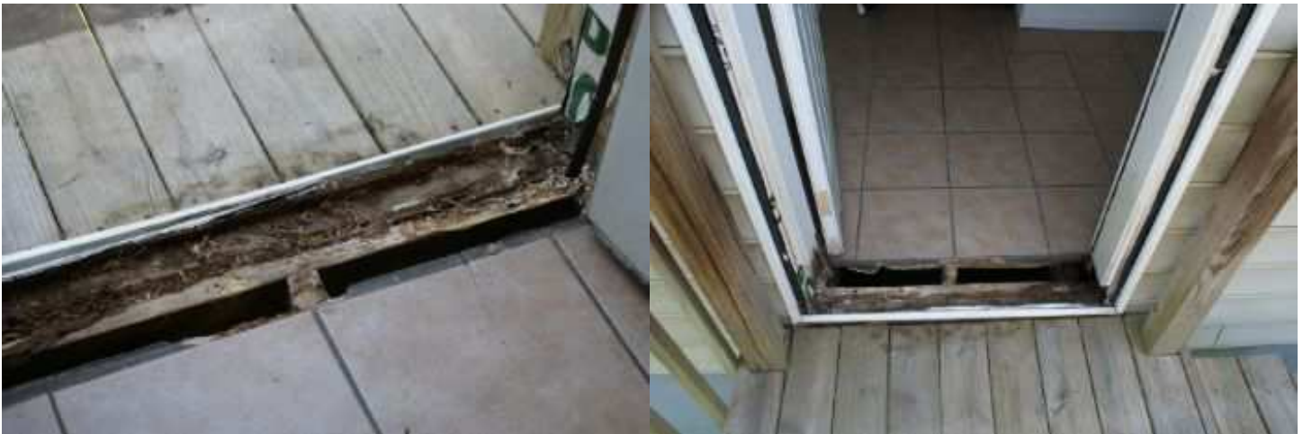
Door needs replacement
