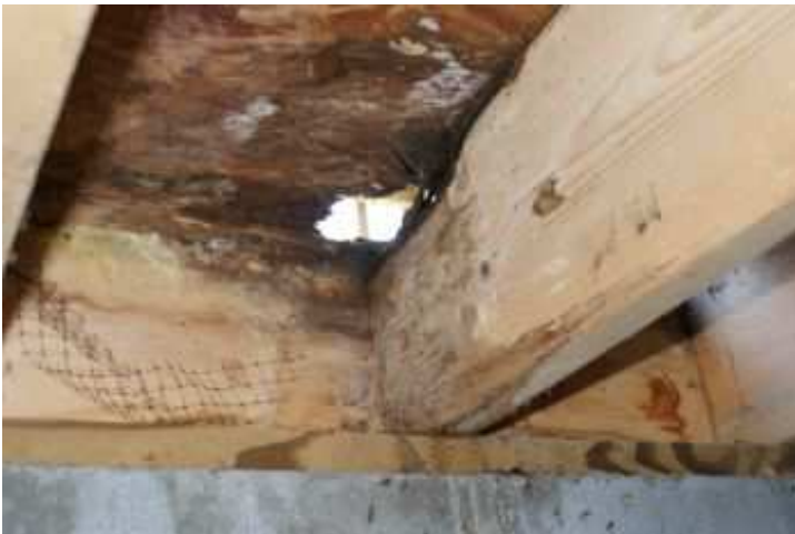
There is a moisture damaged joist under the exterior side door.
