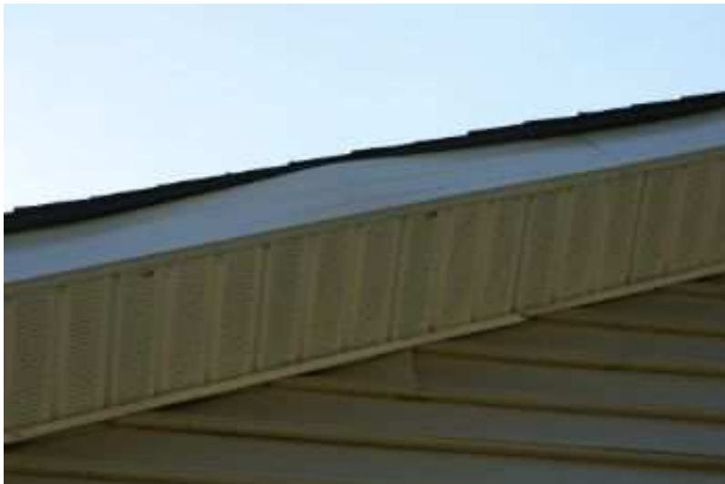
In the rear of house the facial needs to be secured to prevent water intrusion.
