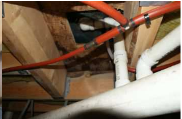
There is evidence of minor sub floor moisture damage under the tub.
