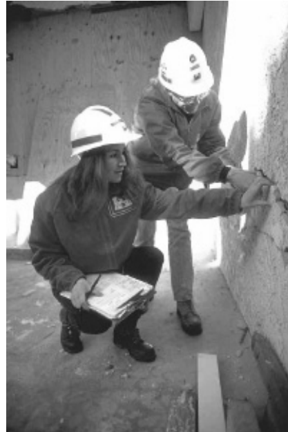
Inspection teams verify damages to public facilities.
