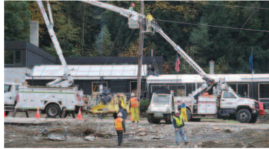
IBEW Local 2320, Manchester, NH, members were lauded for their work restoring vital telecom links after a mas- sive flood.
