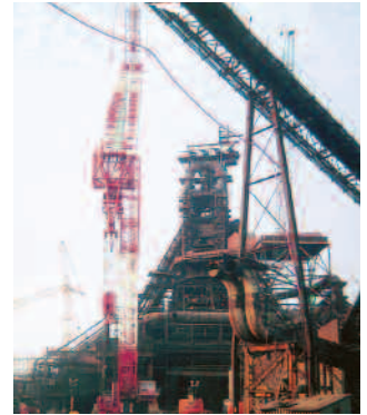
Old #13 blast furnace at U.S. Steel's Gary, IN, works comes down to make way for #14. Meade Electric Co. is the electrical contractor for the project, employing over 200 IBEW Local 697 members and travelers.
