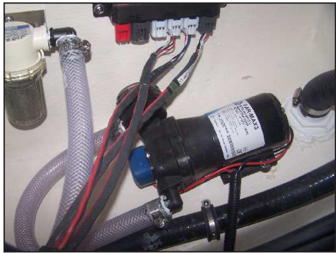
Washdown Pump in Stern Bilge
