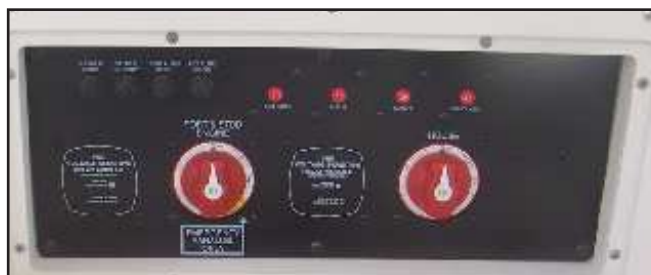
Battery Switch and Breaker Panel
