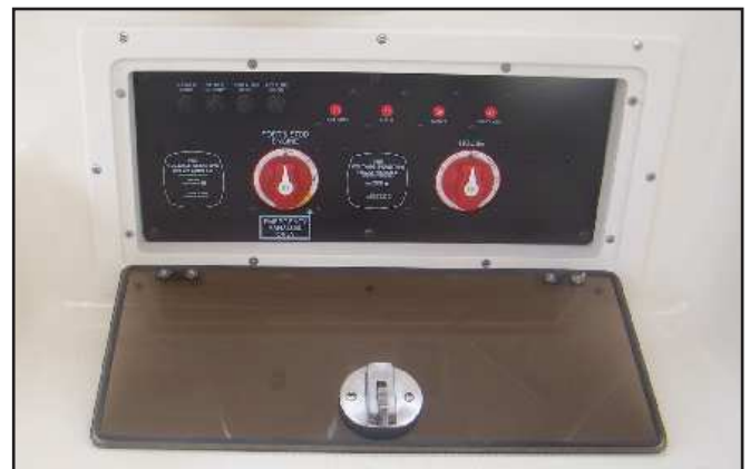
Battery Switches and Circuit Breakers
