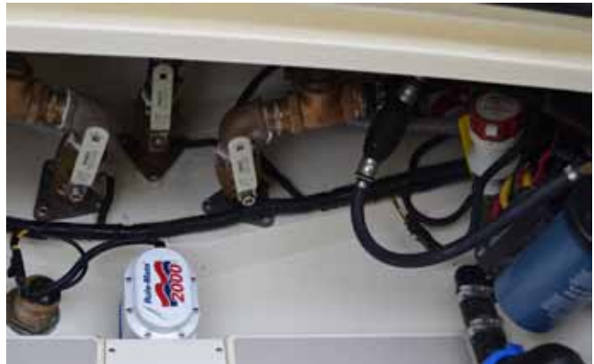
Bilge Pump and Baitwell Pumps
