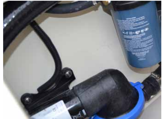
Overboard Discharge Pump in Stern Bilge
