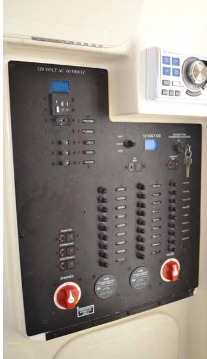
Battery Switches (red)
