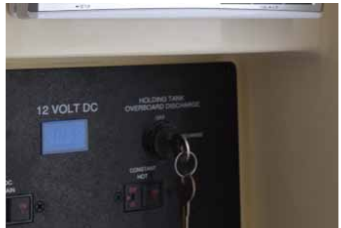
Overboard Discharge Pump Lockout Switch
