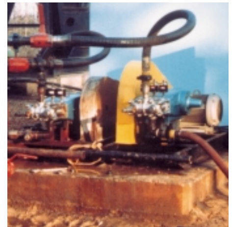
Waste-Water Re-Injection Systems
