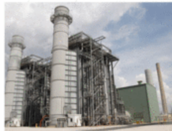
A combined cycle plant
