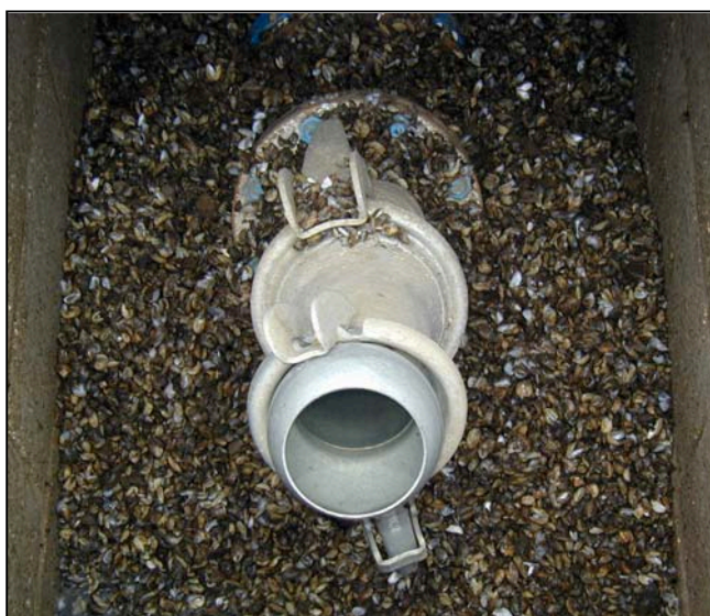
Figure 4.9 Mussels in the drainage chamber of an ozone tank at Walton-on-Thames WTW.
