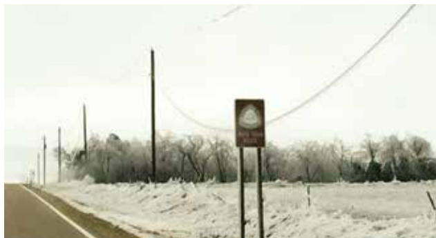
When the temperatures rose on Monday, Nov. 30, another issue arose. Falling ice caused bouncing lines and left 1,665 members without power.
