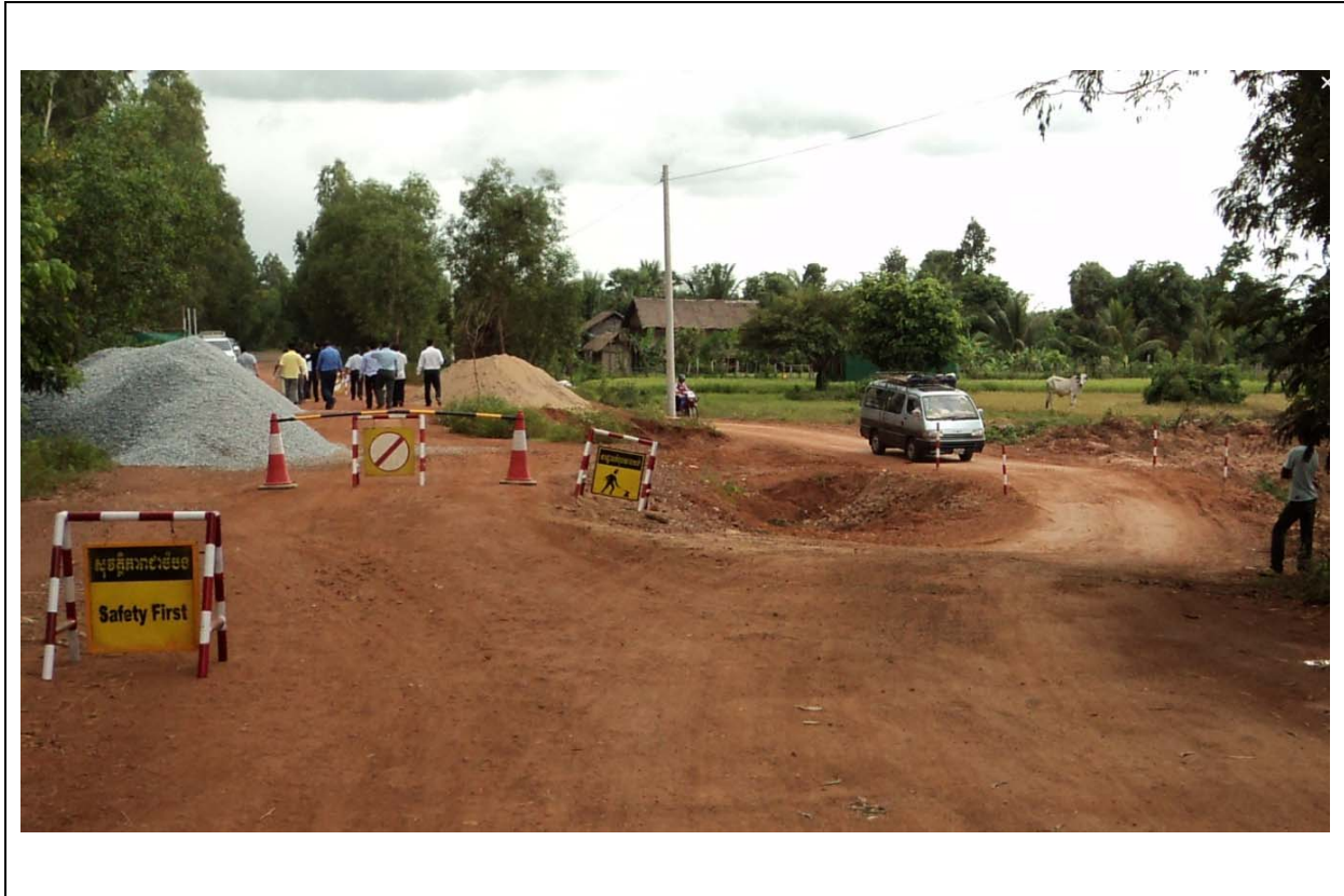
Diversion Road for the RC Box Culvert at PK 16+ 350 SNR65 (Siem Reap)
