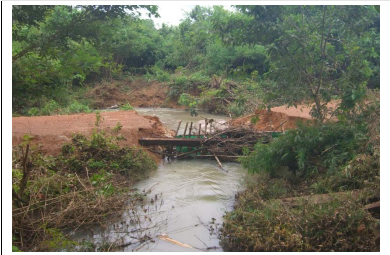
Diversion Road Damaged by Flood (Preah Vihear)
