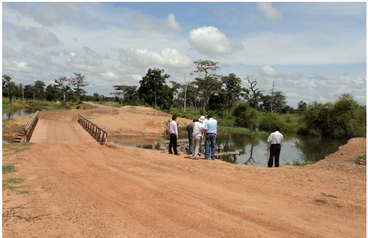
Proposed Location of 2-12.00m Span x 5.00m Wide RC Bridge (Oddar Meanchey)
