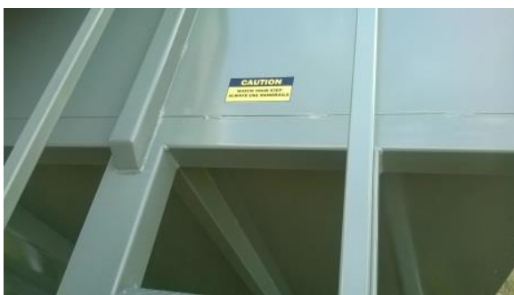
Above Access ladder
