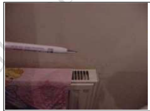
Staining around radiator
