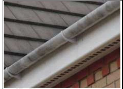
Moss covered gutters
