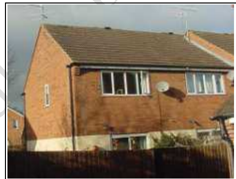
1980's property, cold bridging was found in the lintels
