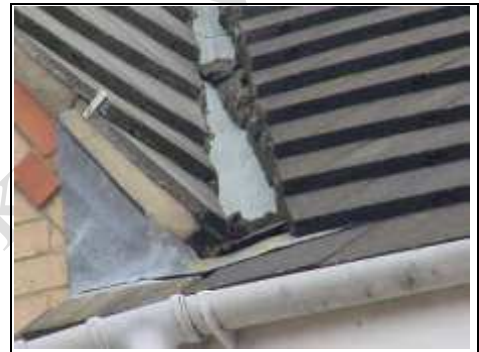
Cement mortar has come away
