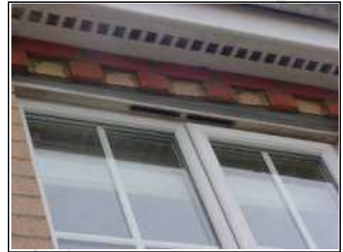
Property not square – twist in lintel
