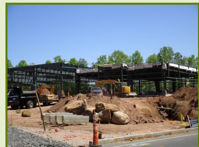
The new GMN USA factory building is well on its way—bringing another business and jobs to Bristol
