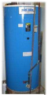
Refrigeration Heat Recovery
