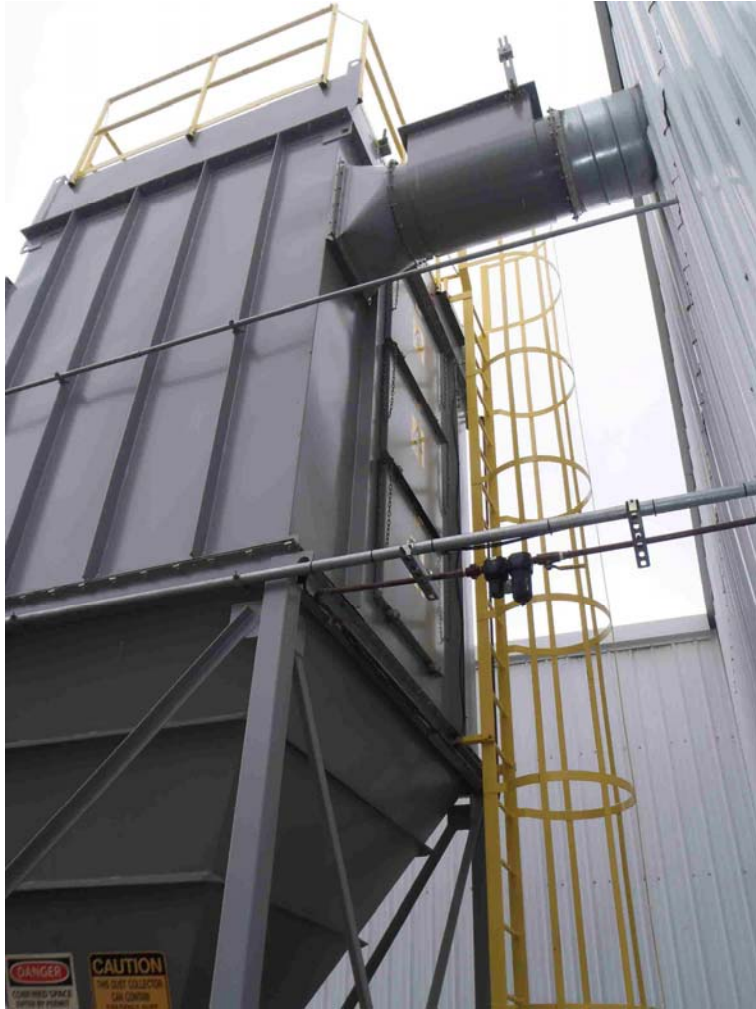
Figure 1 - Rectangular Baghouse pre-Explosion
