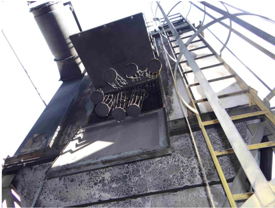
Figure 5 - Bottom Vent Showing Pushed-out Sock Cages
