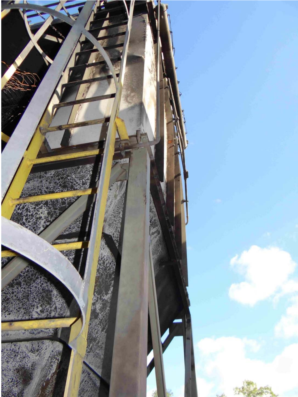
Figure 4 - Side Wall of Collector - Deformation Damage Even Though Reinforced
