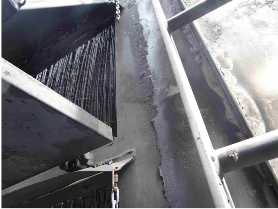
Figure 2 - Close-up of Middle Explosion Panel
