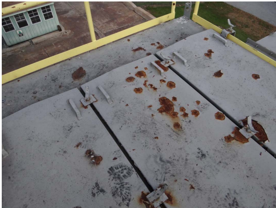
Figure 6 - Top of Dust Collector. Note Deformed Access Doors
