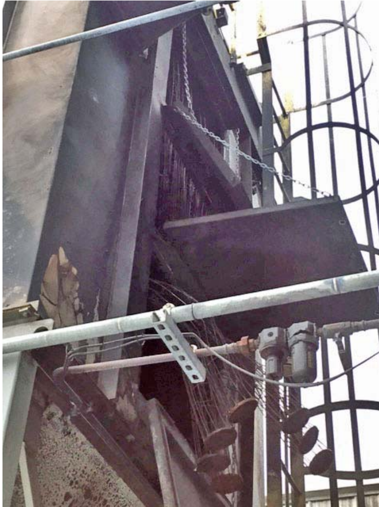
Figure 3 - View of all Three Panels. Note Congestion; Bottom Panel has Sock Cages Pushed out of Opening
