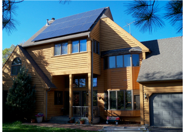
Residential PV solar installation in Minnesota
