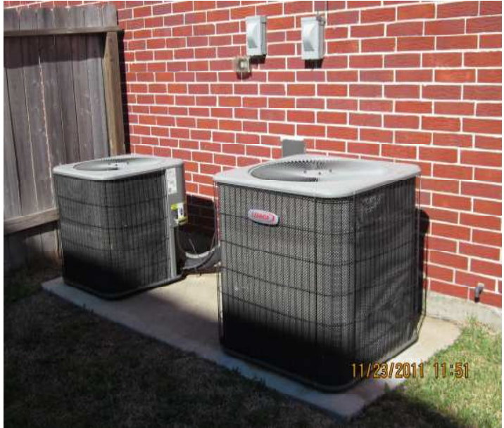
PHOTO NO. 6 TWO A/C UNITS ON SOUTH SIDE
