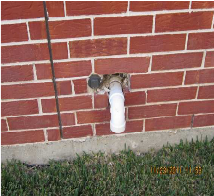
PHOTO NO. 7 NORTH BRICK WALL DAMAGED BY DRAIN
