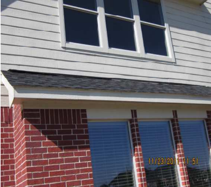
PHOTO NO. 5 DAMAGED ROOF FLASHING AT LOWER BACK ROOF
