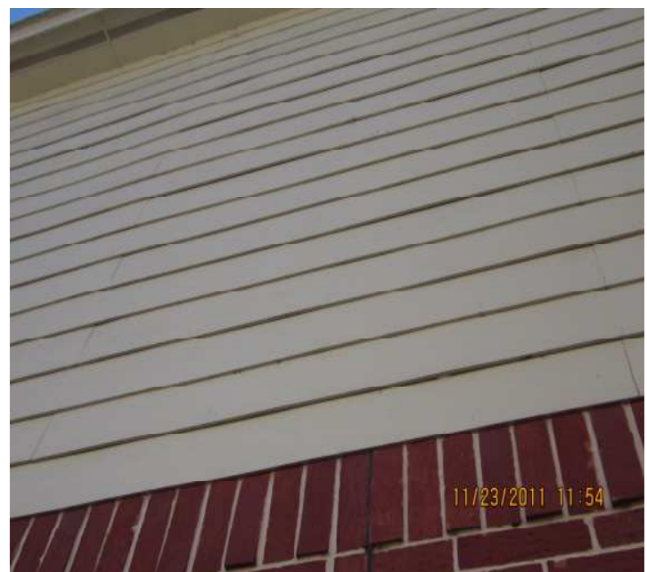
PHOTO NO. 8 GAPS, OPEN SEAMS, AT NORTH SIDE SIDING
