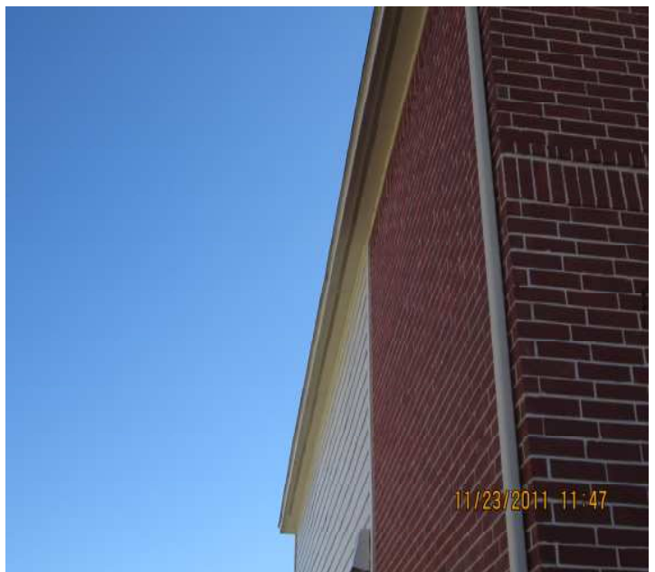
MISSING GUTTERS ON EAST EAVE
