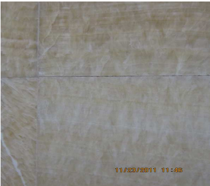
CRACKS IN TILE FLOOR GROUT IN ENTRYWAY
