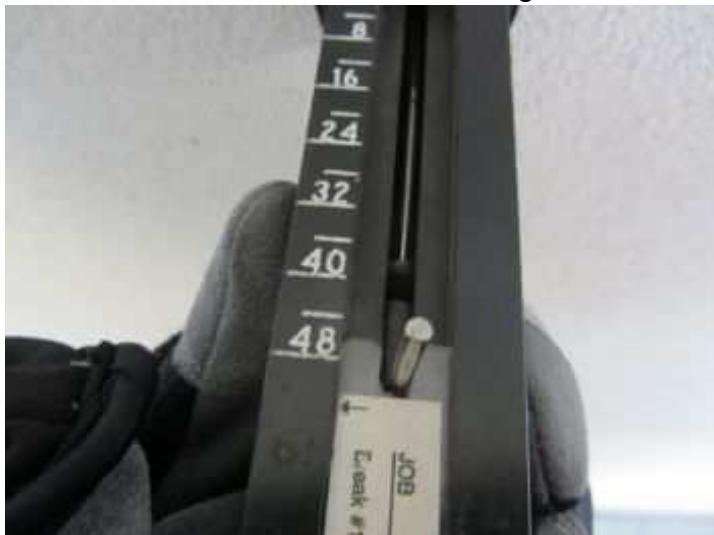
Tests with the Structure Resistance Tester (SRT) was 48 pounds of resistance without any penetration into the wood.
