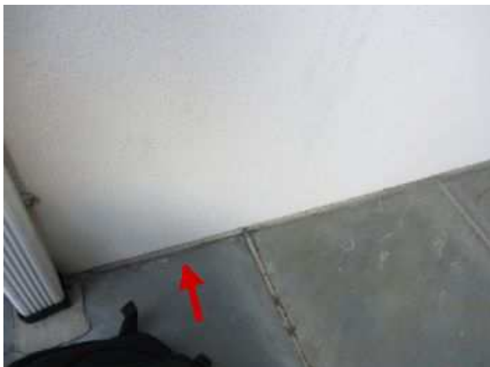
The EIFS is in contact with concrete the system should be at least 2 inches about grade. Water can wick its way into the siding material. This will result in deterioration of the siding material.
