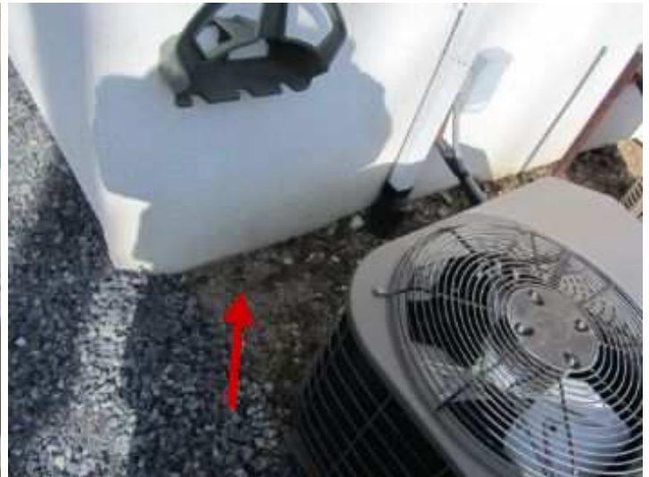
Although the External Insulated Finish System (EIFS) was improperly installed, the system appears to be in acceptable condition, with the exception of the following areas. At a minimum, we recommend having a licensed EIFS contractor make the repairs as noted in each of the following: 1) Below grade terminations of EIFS it should always terminated above grade a minimum of 6 to 8 inches of clearance. The terminating below grade can allow moisture to wick up behind the system. This also creates conditions conducive to termites and carpenter ant infestations.
