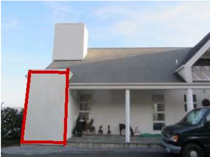
Small part of the wall had front elevated moisture levels, and the wood substrated has been damage by moisture needs to be replaced.
