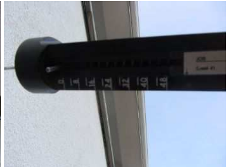
Tests with the Structure Resistance Tester (SRT) was 48 pounds of resistance without any penetration into the wood.
