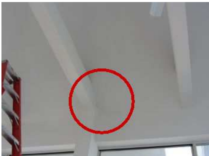
There are two areas on the ceiling where cold spots were detected with the thermal infrared camera, check with moisture meter reading were 5% moisture no moisture present in the cold spots on the ceiling.
