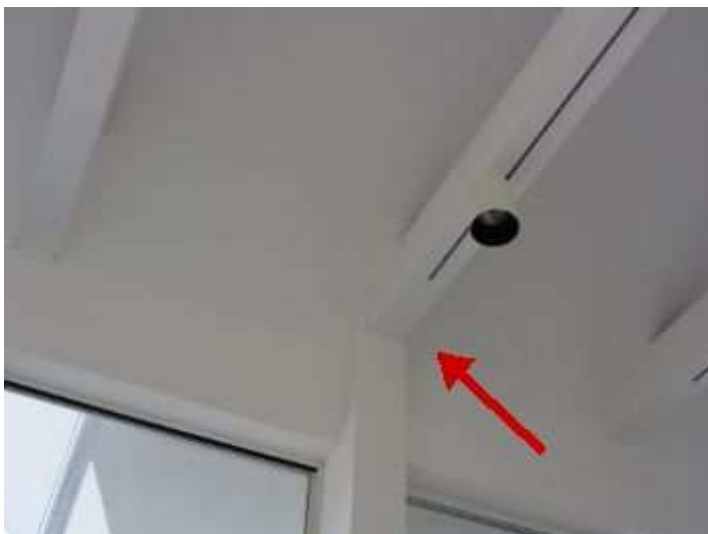
There are two areas on the ceiling where cold spots were detected with the thermal infrared camera, check with moisture meter reading were 5% moisture no moisture present in the cold spots on the ceiling.
