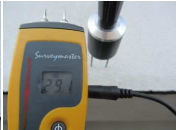
GE Surveymaster moisture meter probe reading between 29.1% to 39.7% moisture
