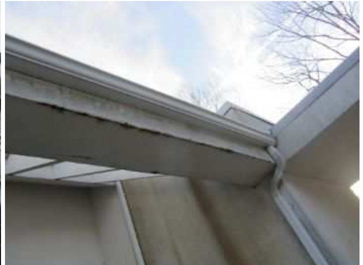
The Inspector recommends to apply AllGuard Silicone Elastomeric Coating or a another Masonry Water proofing sealant to this exterior masonry wall to protect it from moisture entering and help make it watertight.
