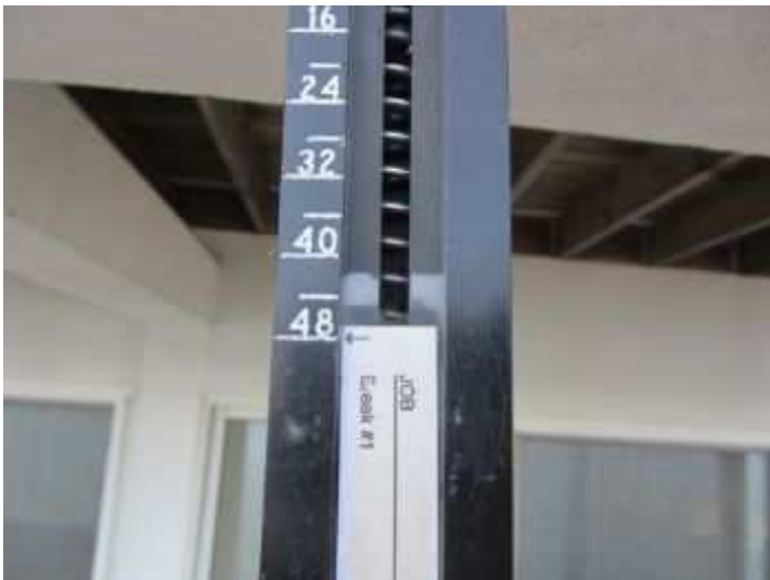
Tests with the Structure Resistance Tester (SRT) was 48 pounds of resistance without any penetration into the wood.
