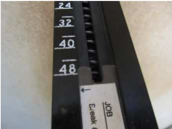
Tests with the Structure Resistance Tester (SRT) was 48 pounds of resistance without any penetration into the wood.
