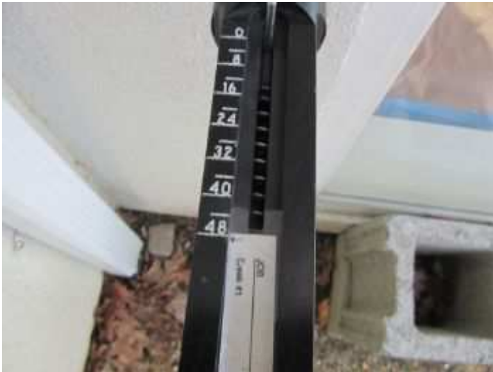
Tests with the Structure Resistance Tester (SRT) was 48 pounds of resistance without any penetration into the wood.
