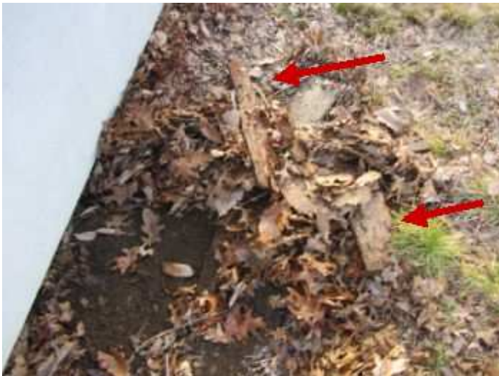
Wood behind the garage should be removed because it is a conducive conditions for termites.
